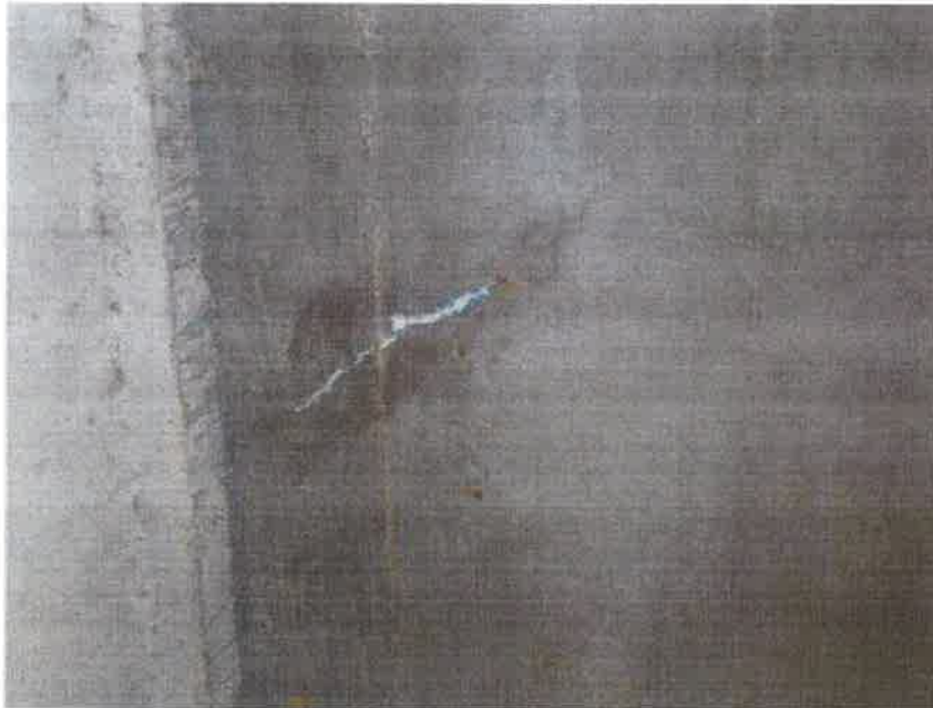
Photo Number: 3 Photo Taken: 07/21/2023 DIAGONAL CRACKING WITH EFFLORESCENCE AT SOUTHWEST CORNER UNDERSIDE
